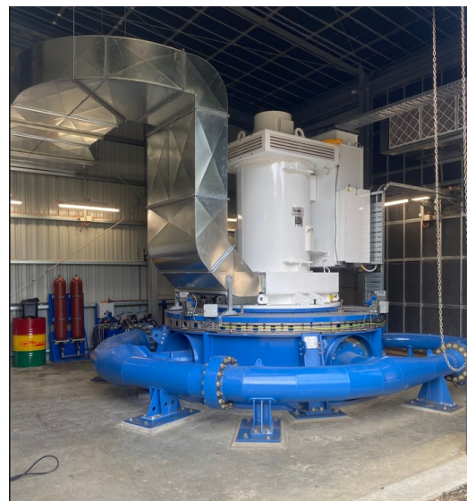
Scottsdale Power Station turbine
