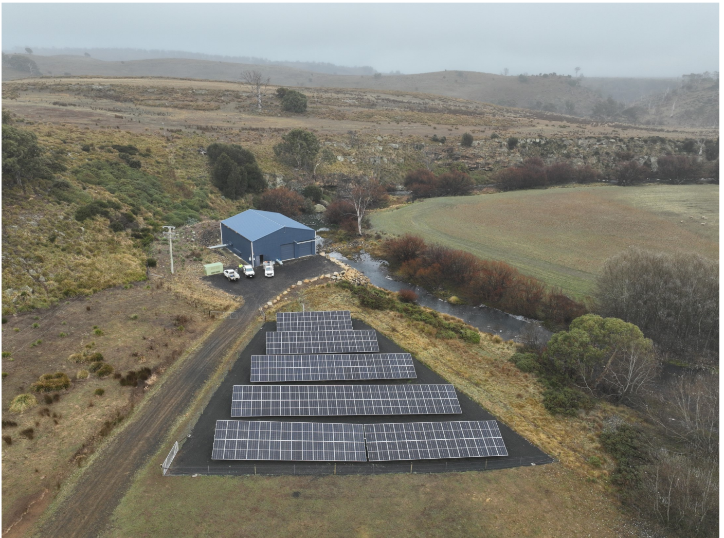
Solar array installation at the Shannon River pump station on the Southern Highlands Irrigation Scheme
