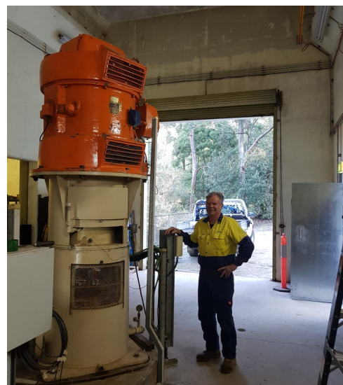
Bill with the Sassafras Wesley Vale Irrigation Scheme Great Bend pump, which has been in service since 1968.
