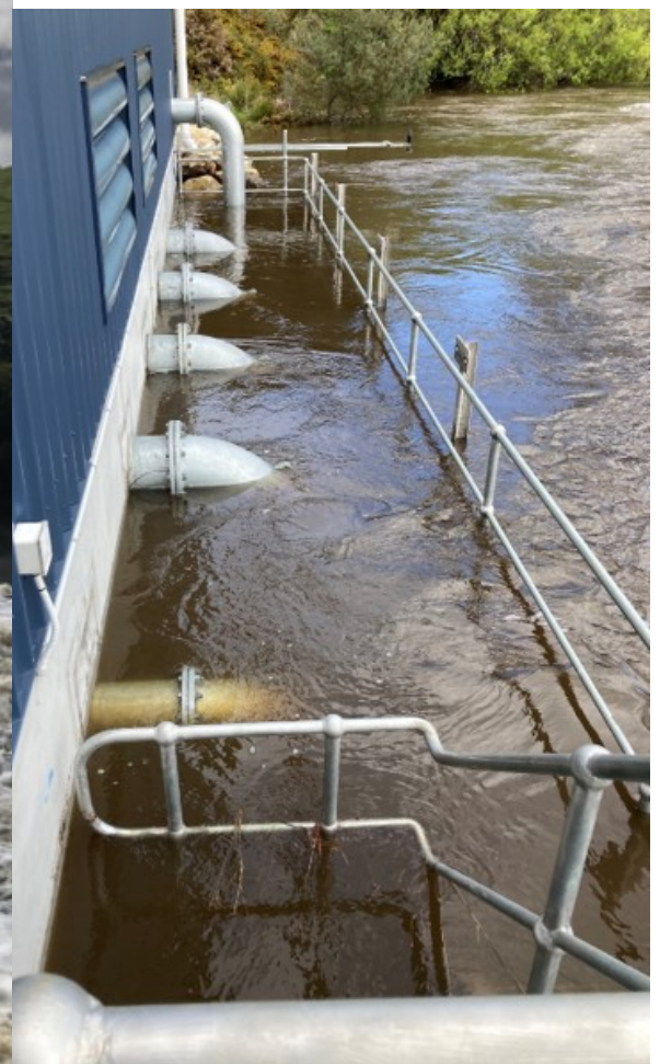
Shannon River Pump Station in flood ↑
