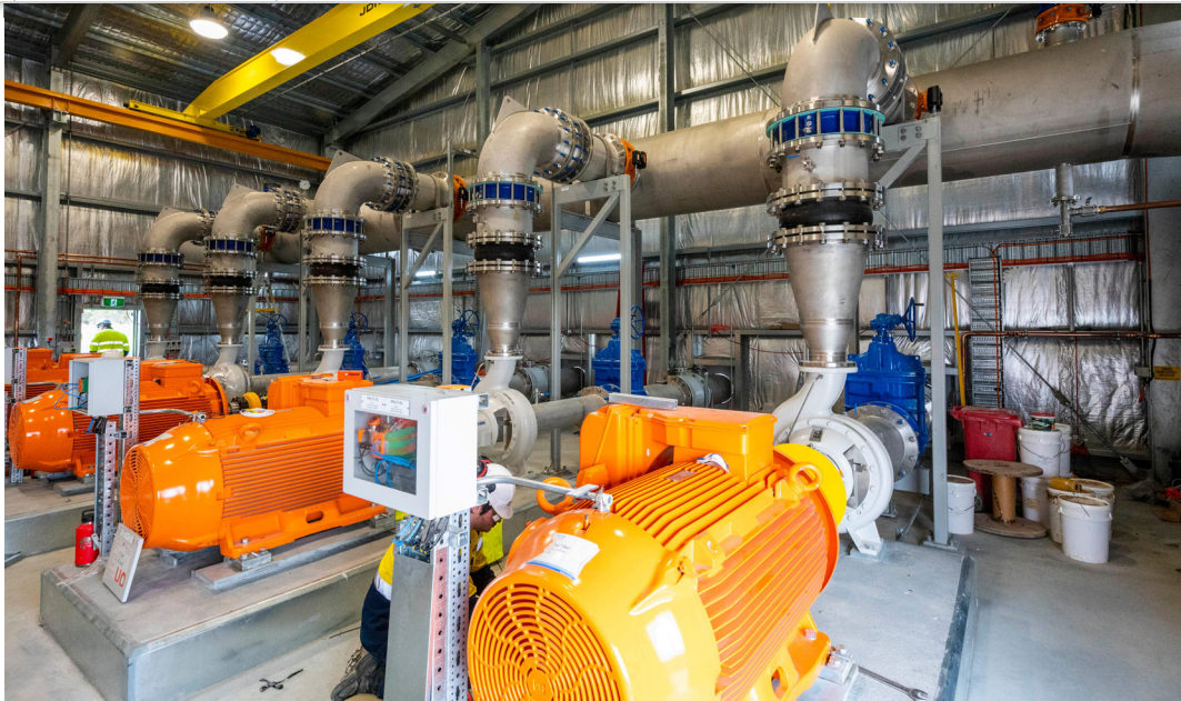
Figure 1 - Poatina Pump Station
